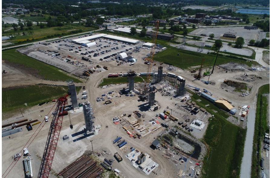
A look at the side span piers and anchor piers on the Canadian bridge site.
