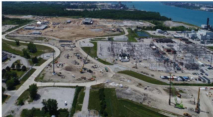
Workers are building up the foundations for the approach bridge span piers.
