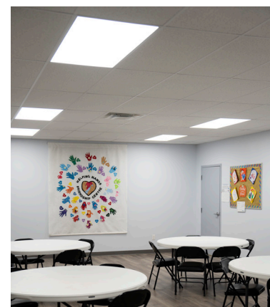
A new drop-down ceiling at the Helping Hands Friendship Centre provides a comfortable space for participants.
